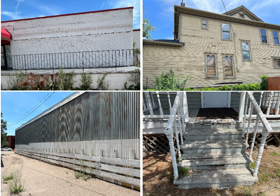
Figure 2. Deteriorated Exterior Finishes and Stairways
