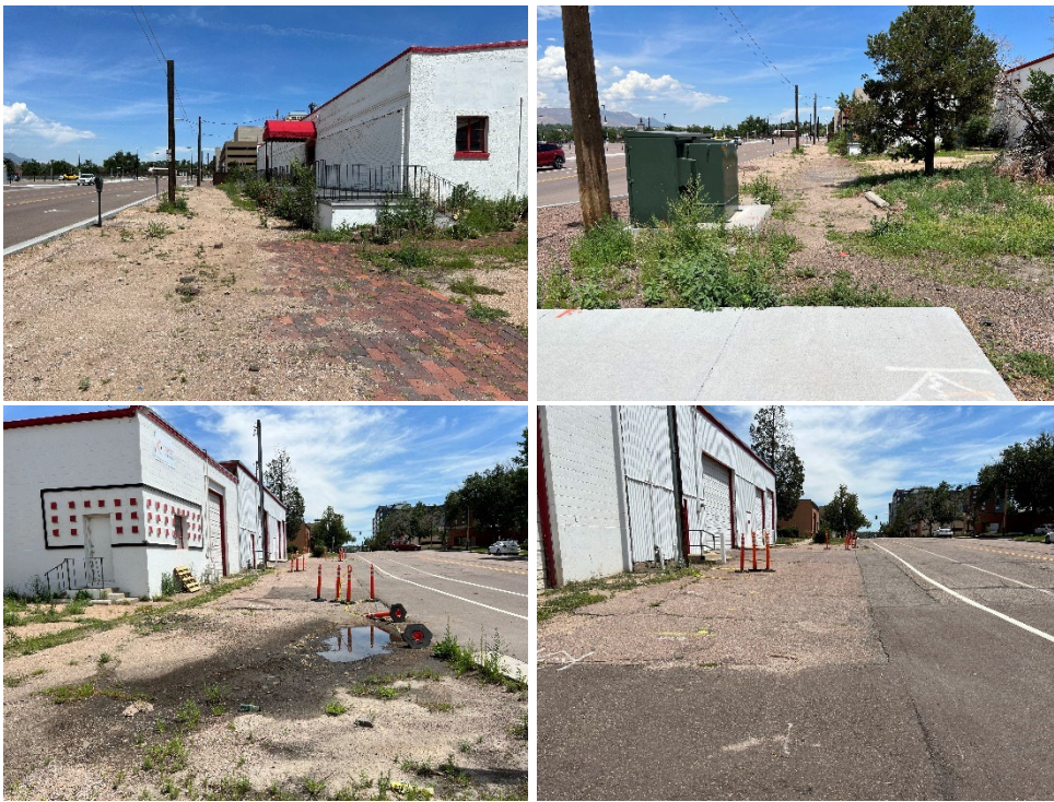
Figure 3. Poor Provision of Street Improvements for Pedestrians
