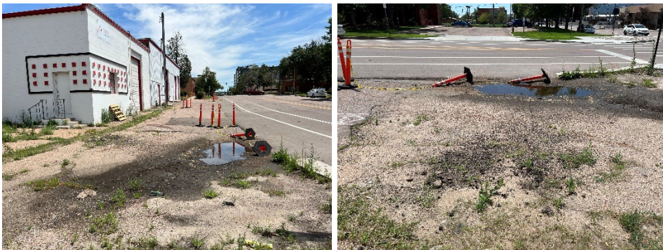
Figure 9. Evidence of Standing Water
