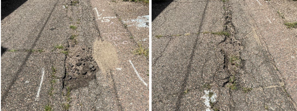
Figure 4. Poor Provision of Street Improvements for Vehicles
