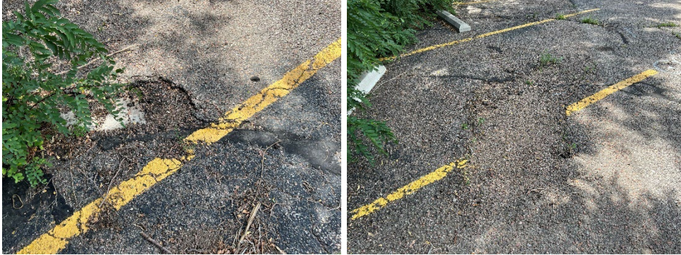
Figure 10. Deteriorated On-Site Parking Surfaces
