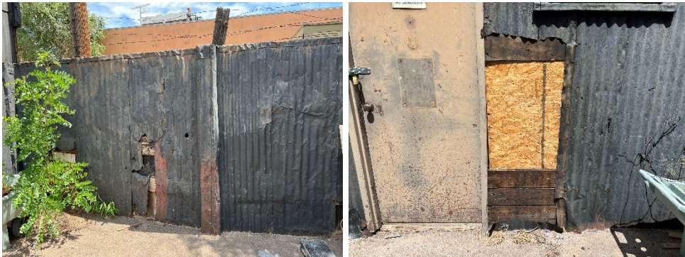
Figure 12. Deteriorated Fences and Walls
