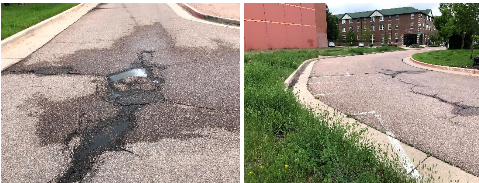
Figure 2. Poor Provision of Street Improvements
