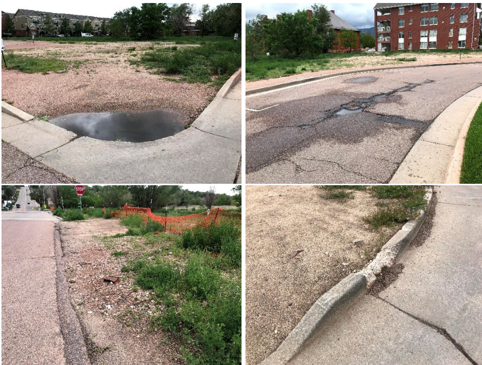
Figure 9. Deteriorated Pavement and Curbs and Missing Sidewalks
