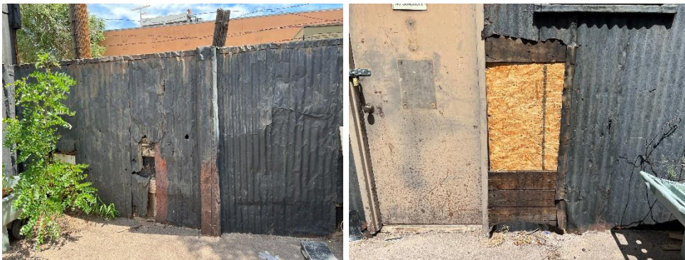
Figure 12. Deteriorated Fences and Walls
