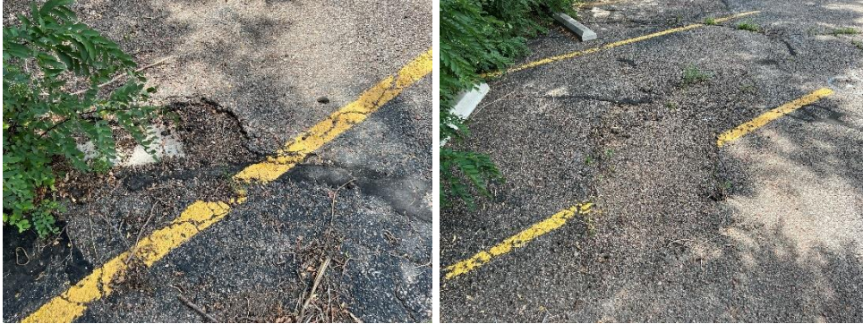
Figure 10. Deteriorated On-Site Parking Surfaces
